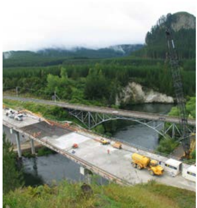
THE NEW SH1 BRIDGE AT ATIAMURI UNDER CONSTRUCTION IN 2013. In partnership with NZTA, Raukawa were heavily engaged in the project to replace the old bridge at Atiamuri.
